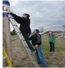
Garette Byron inserts and tightens the screws to perfection. He likes to work as close to the ground as possible! Cooper sorted and handed up the fasteners.
